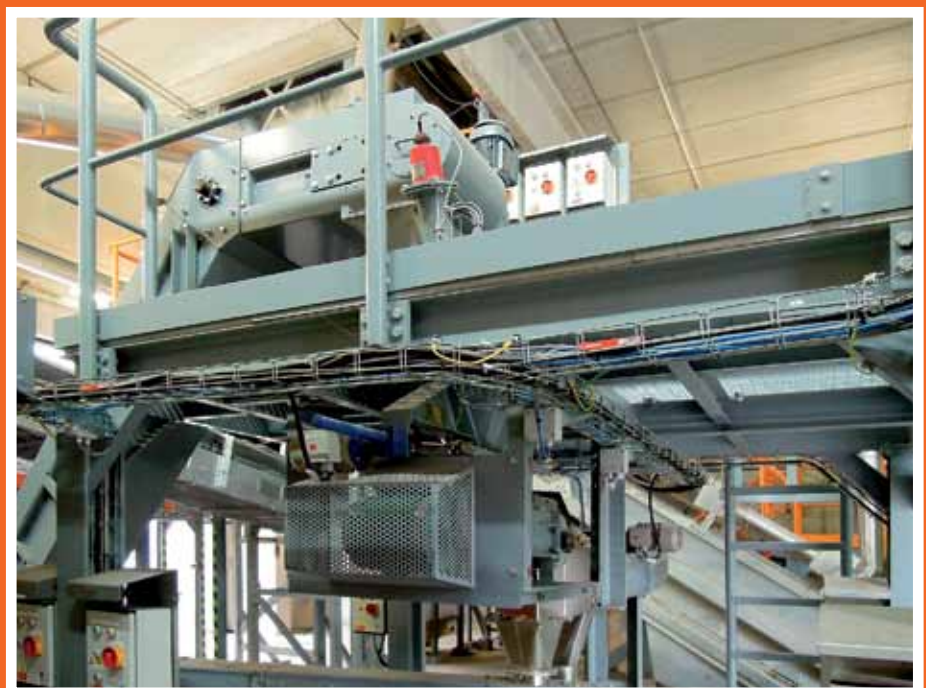
Newly installed sampling station of SAF - The inclined belt outlet to the homogenizer
