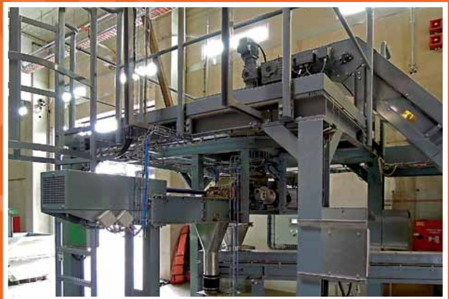
Newly installed sampling station of SAF - Distributing system under the homogenizer
